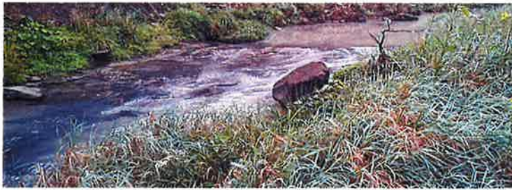
Figure 24 — Fourmile Run upstream from Salt Springs Rd. (RM 0.7) September 2013. Perpetual turbidity emanating from the Mahoning Valley Race Course construction site degraded habitat quality in Fourmile Run and in the Mahoning River.
