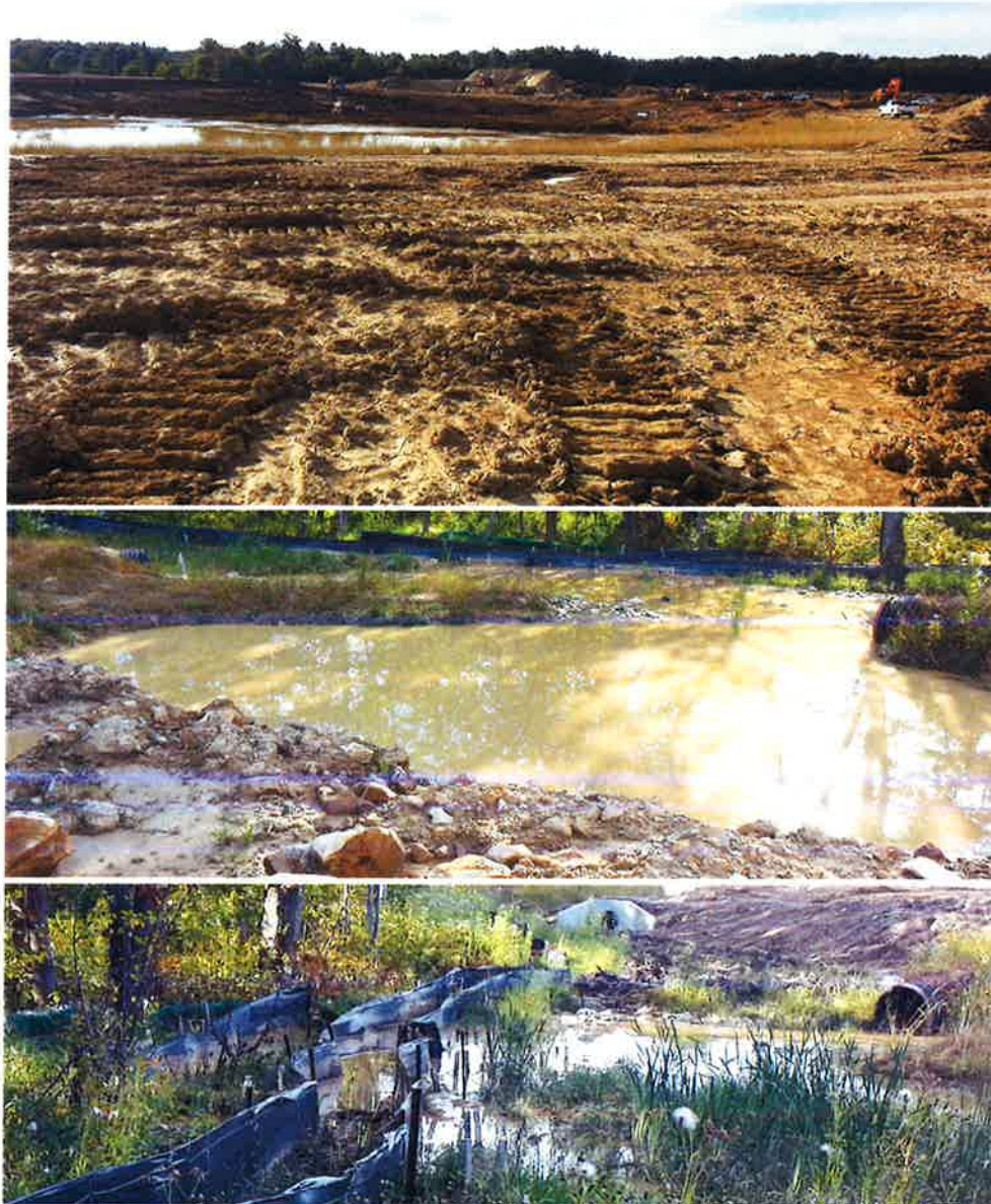
Figure 25 — The Mahoning Valley Race Course construction site, September 2013. Turbidity in Fourmile Run and the Mahoning River were attributed to this location. A day before the photographs were taken, the large basin in the upper photo had been pumped out, overtopping the silt fence in the lower photos.
